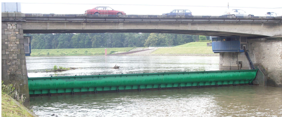
Fig. 5. The flap of weir after exchanging, view from the side of tail water
