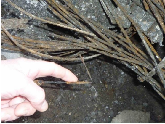
Fig. 5a. Corroded wire pulled out from the duct.
