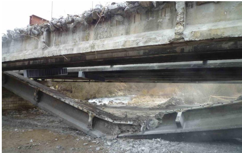
Fig. 5c. Falling down girder during demolition works.
