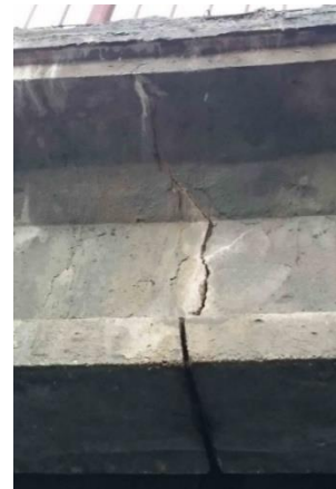
Fig. 4b. Detail of the primary crack.
