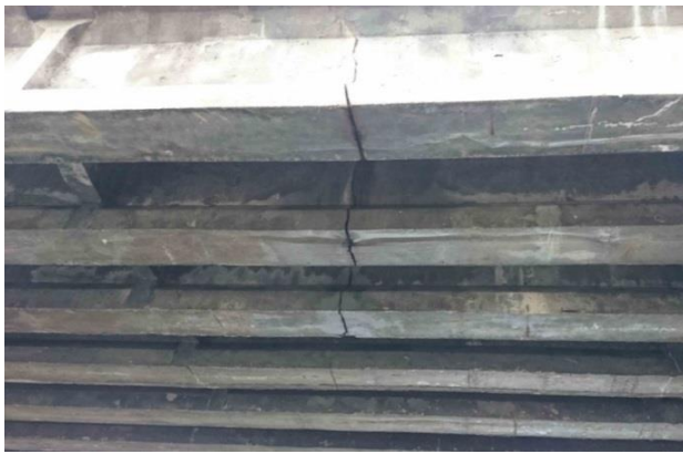
Fig. 4a. Brittle failure on the 4 edge girders.
